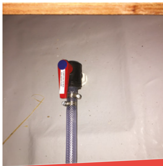
Seawater intake valve
