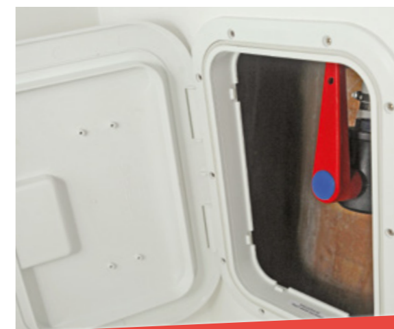
2 Seawater intake valve
